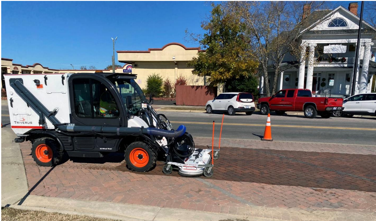
Figure 15. Cleaning PICP in Fayetteville, NC. The installation had not received regular cleaning. Equipment was used to remove accumulated sediment from the joints.
